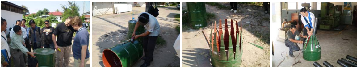
Figure 2 Fuel feeder cone is made of used oil drum
