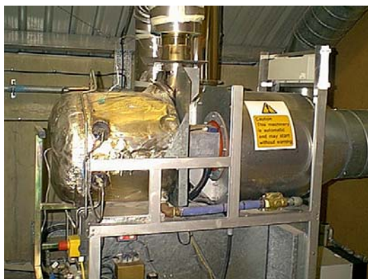
Figure 3 Capstone CHP operating on biogas
