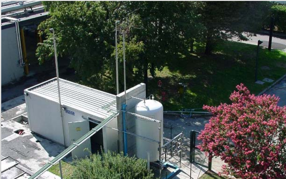
4 m 3 Hydrogen at 10 bar Connected to the Hydrogen network
