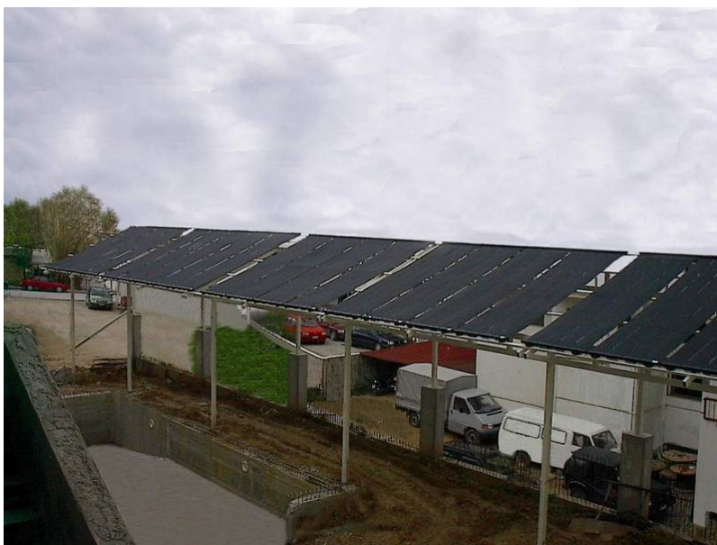
Figure 10: Solar polypropylene collectors for swimming pool heating
