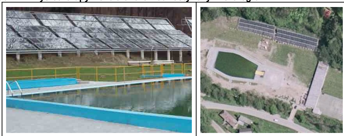
Figure 1: Solar system on outdoor swimming pool at Rusava, left: western part of the collector area (© Czech RE Agency, o.p.s.), right: satellite view, collectors on upper part (© www.geodis.cz, © mapy.seznam.cz)
