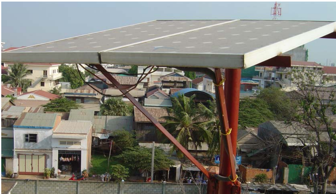
Figure 4 PV panel on the fixed stand on ITC roof
