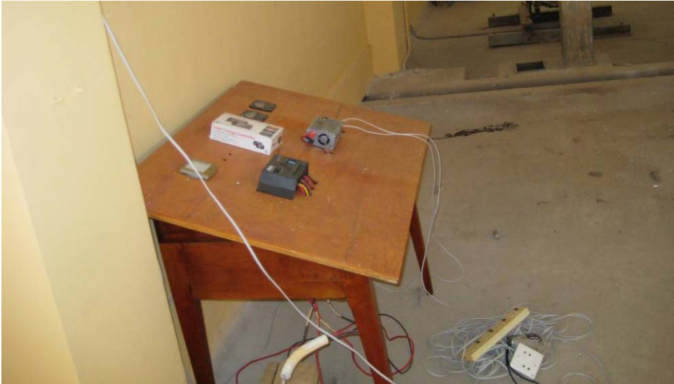
Figure 5 Charge controller and Inverter
