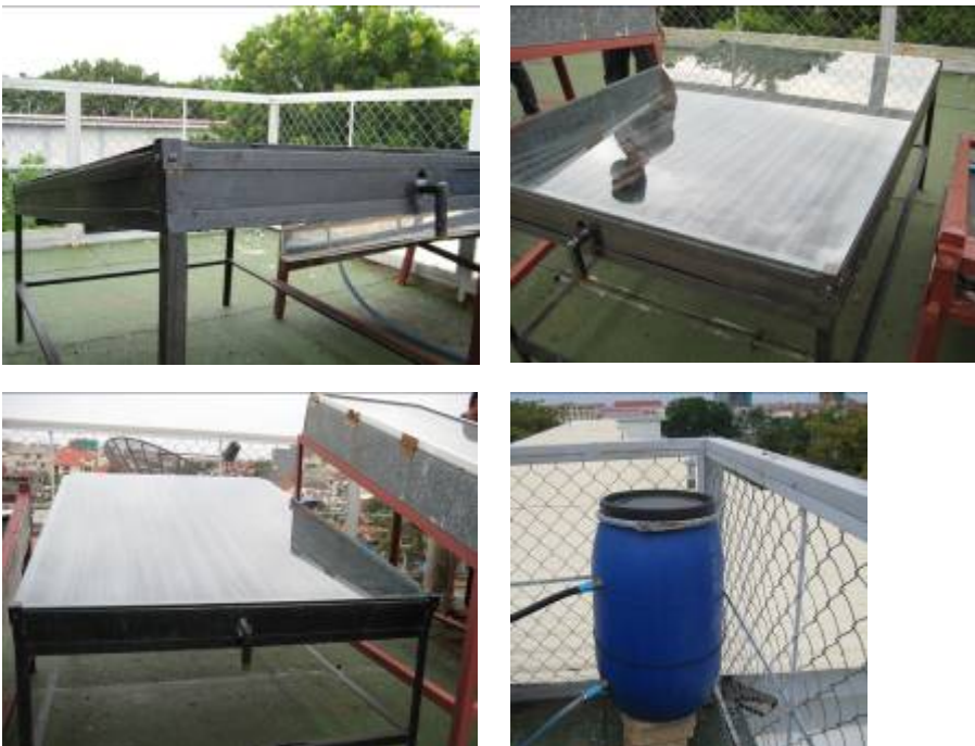
Figure 6 Solar Hot Water
