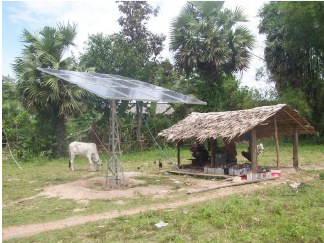
Figure 3: Battery Charge Station in Kor Village
