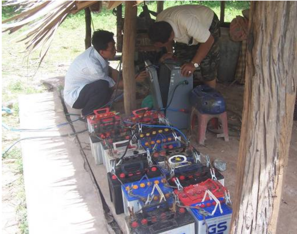
Figure 4: Charge Controller Box for Battery Charge Station in Kor Village
