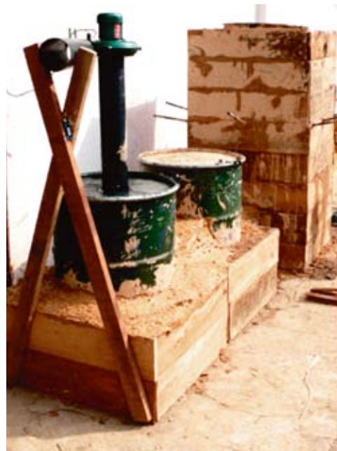
Wood gas generator with gas cooler and attached fan
