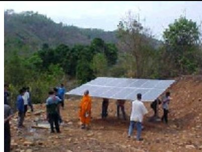
The solar PV system in the village
