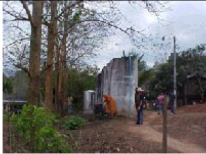
The water storage system in the village
