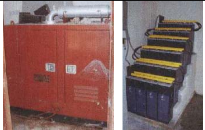
Genset and battery bank
