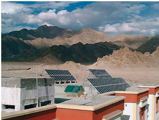
Figure 3: Off grid Solar system (Source SMA)
