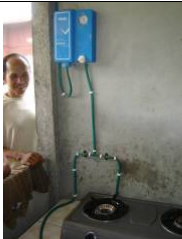
Biogas cooker with gas pipeline and pressure measurement device
